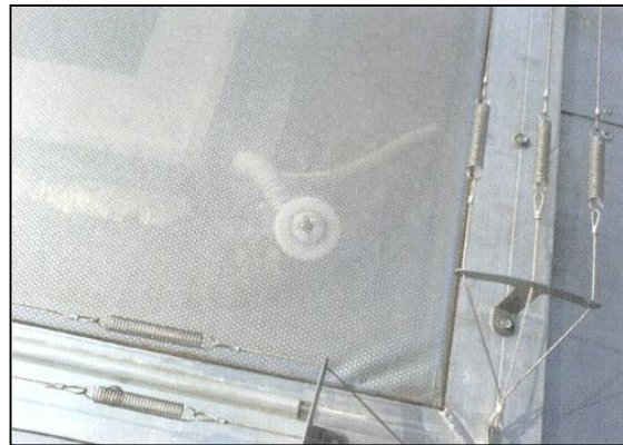
Figure 2.4: Detail of the framing and wires that protect the material from birds puncturing the cushions (LeCuyer et al. , 2008)
