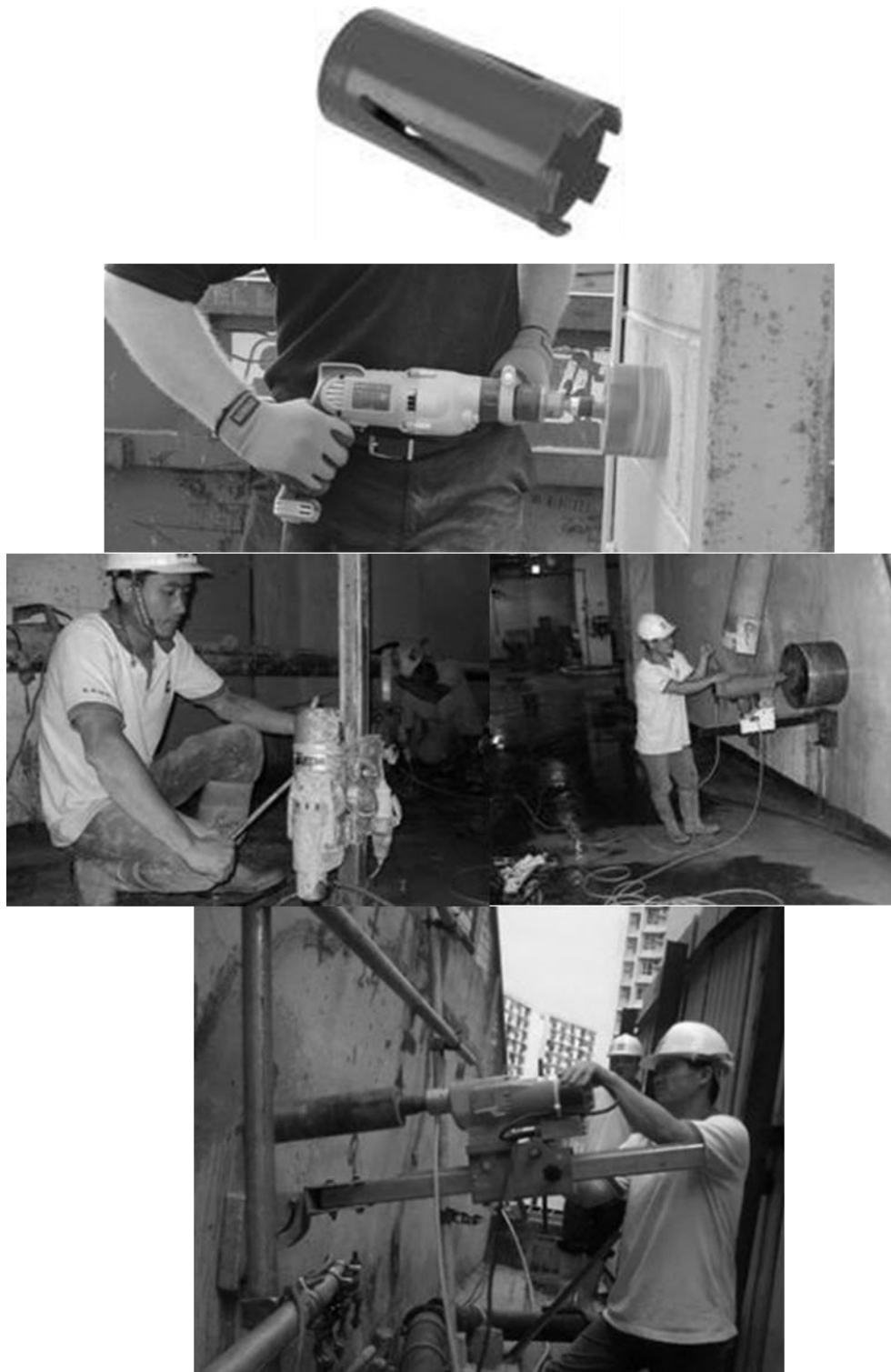
Figure 149 Diamond boring drill equipment and application to core extraction (source: first two from Toolstop, 2013 and the others from China Flying Technology Ltd., 2013)
