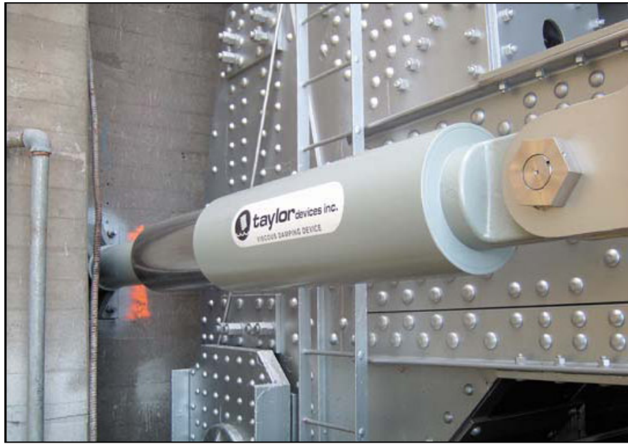
Figure 1.3 Fluid damper installed in a building [15]
