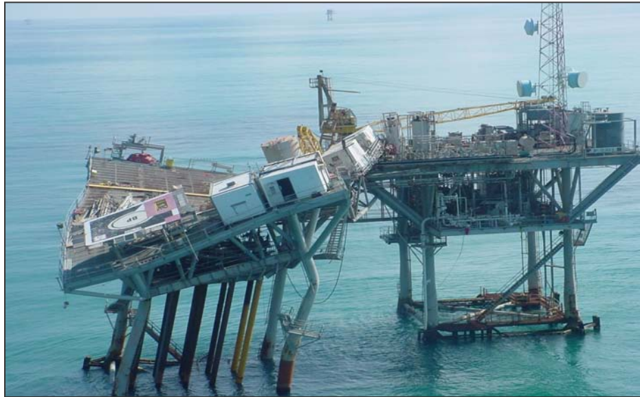
Figure 2.1 Oil station damaged by high speed wind [Mc.Carthy Building Company records, USA]
