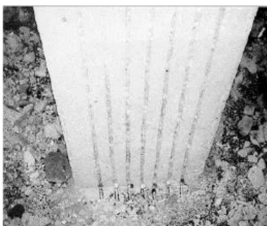
Strengthening of a column with NSM FRP rods (Alkhrdaji et al. 1999, cited by De Lorenzis (2002))
