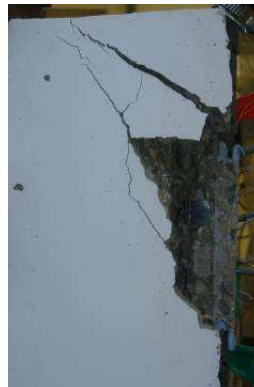
Figure 3.4 - Cone-type failure in the concrete in specimen 1-2[C12/60/S/3.2p]
