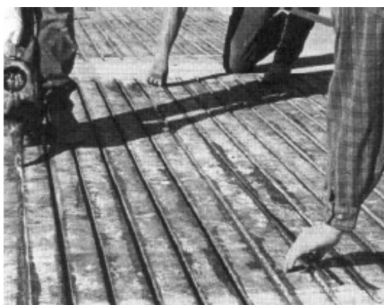
Strengthening of negative moment regions of a bridge deck with NSM FRP bars (Parretti and Nanni, 2004)
