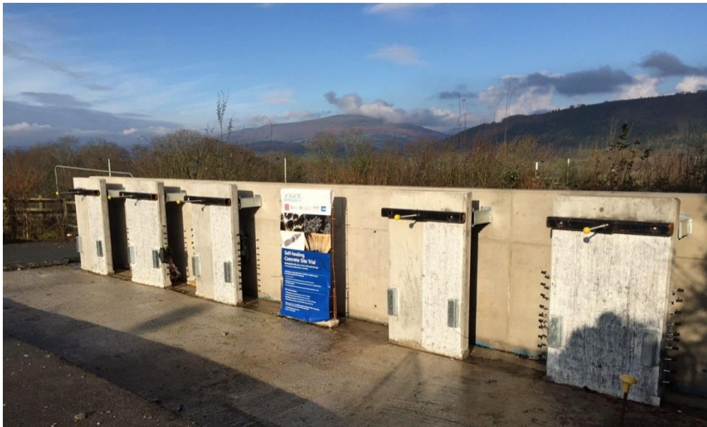
Figure 8.27: The five panels cast. The bacteria-based self-healing concrete panel is the third from the left.
