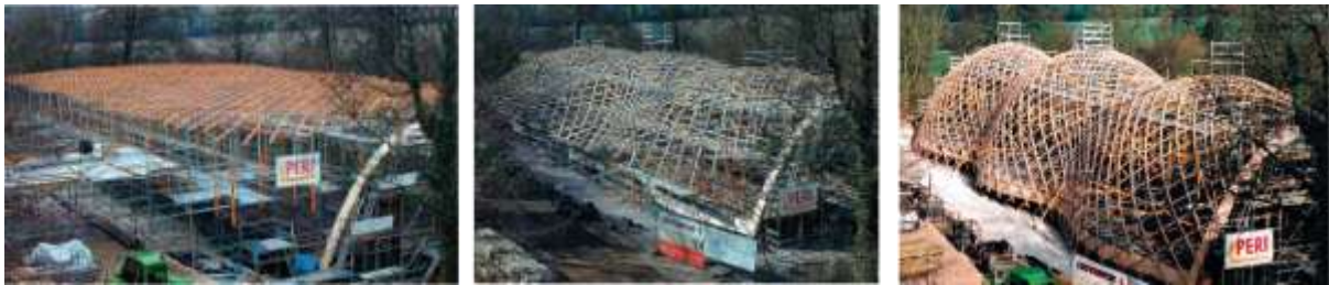
Figure 1. 24 Weald and Downland gridshell construction. Lowering into shape. (Harris et al. , 2003a) p32
