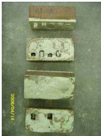
(c) Example of combined failure ('Tradesman Sandfaced (Atlas)' brick)
