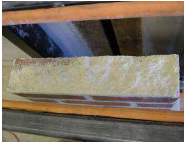
(c) Mortar joint failure
