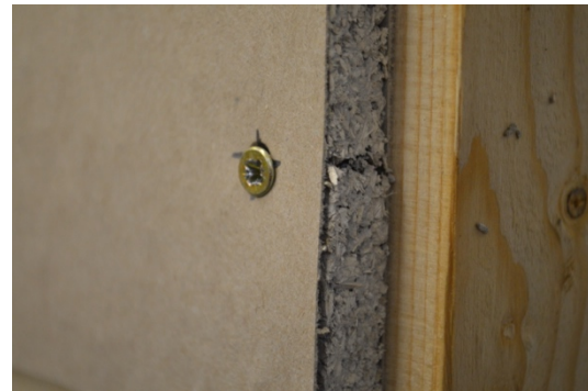
Figure 3 Breathaboard Localised Splitting Failure
