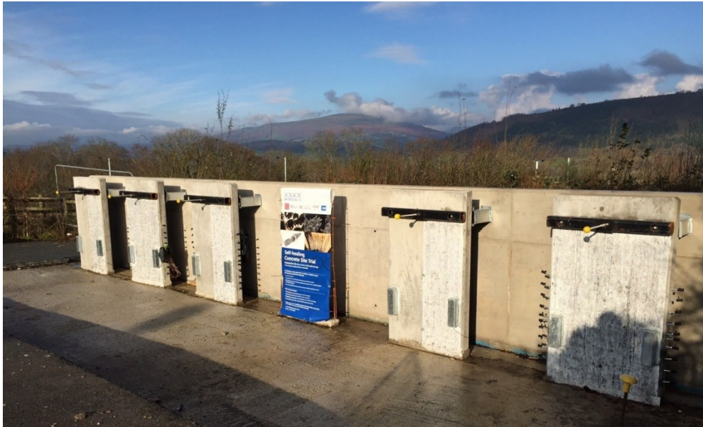
Figure 4 The five panels cast. The bacteria-based self-healing concrete panel is the third from the left.
