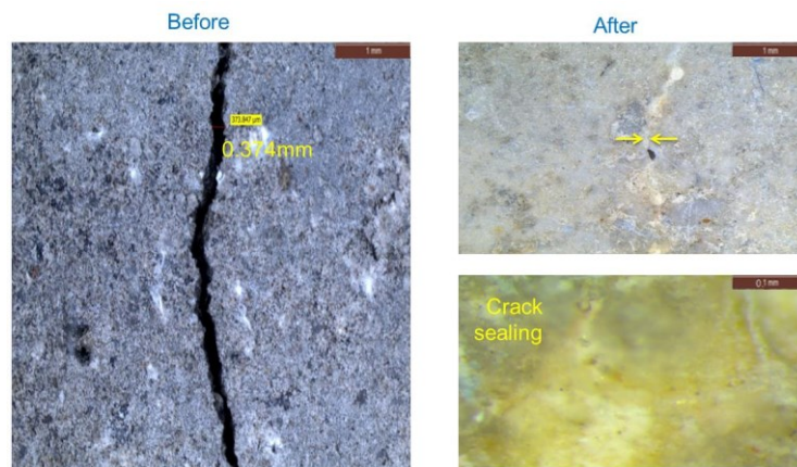
Figure 1 Precipitation of calcite in a crack as a result of bacterial conversion of calcium acetate [5]
