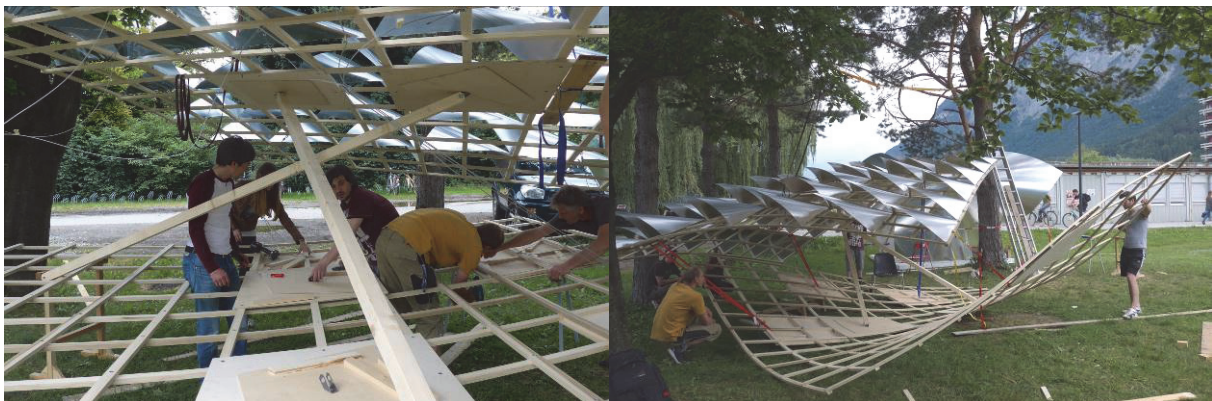
Figure 6: Two struts connected to both lattice grids by full swivel - connection detail (left) and lattice grids were brought into their predefined position by the means of lashing straps (right)
