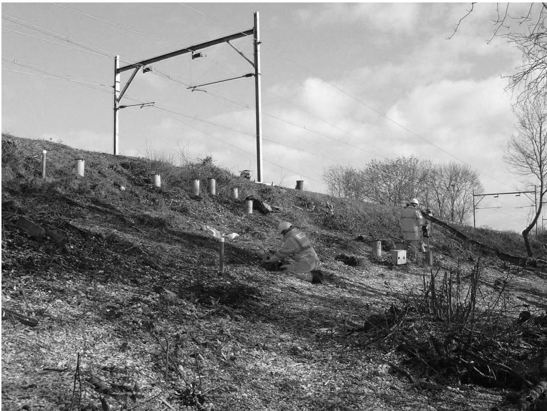
Figure 2: Photograph showing the south side of the embankment in March 2010, shortly after the second vegetation clearance.
