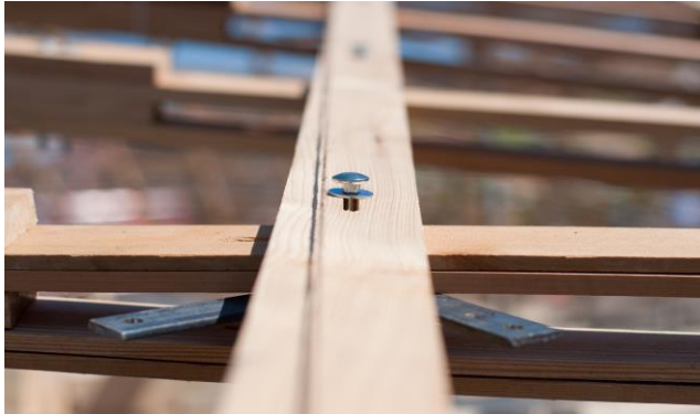
Figure 2.13: Pavilion ZA: typical connection showing thinner laths used for higher curvature areas at entrances, slotted hole and steel bracket for bracing attachment (image – AStA Cluj)
