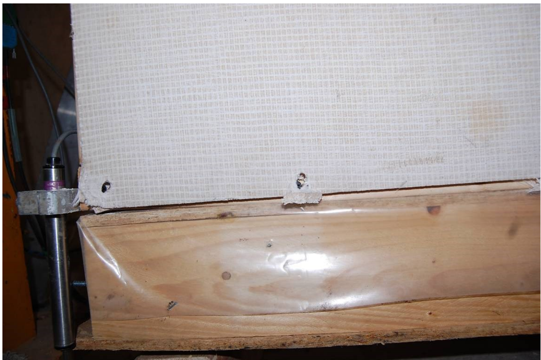
Figure 10 Screws pulling through sheathing board
