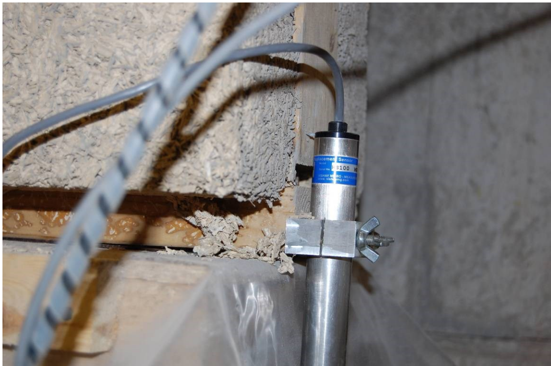
Figure 8 Leading stud connection failure
