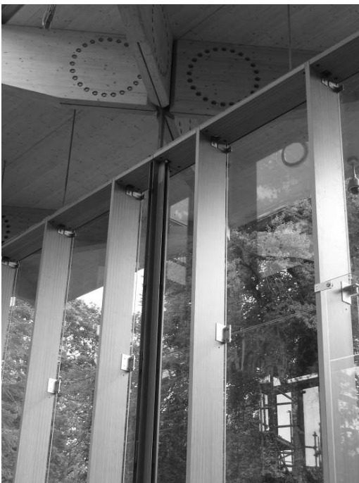
Figure 13: Glazing mullions, showing the detailing that maintains visual expression of the steel column and timber structure (Image copyright: Buro Happold)
