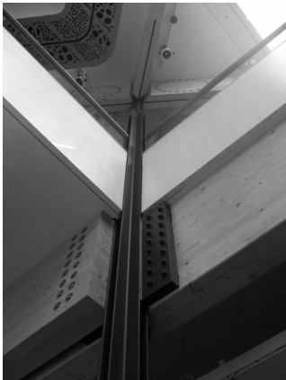
Figure 7: Column flitch plate connection detail at the corner of the atrium (Image copyright: Buro Happold)
