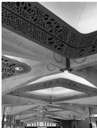
Figure 16: Completed roof structure showing suspended modular lighting/acoustic panels decorated with patterns of the microscopic images of cellulose (Image copyright: Buro Happold)
