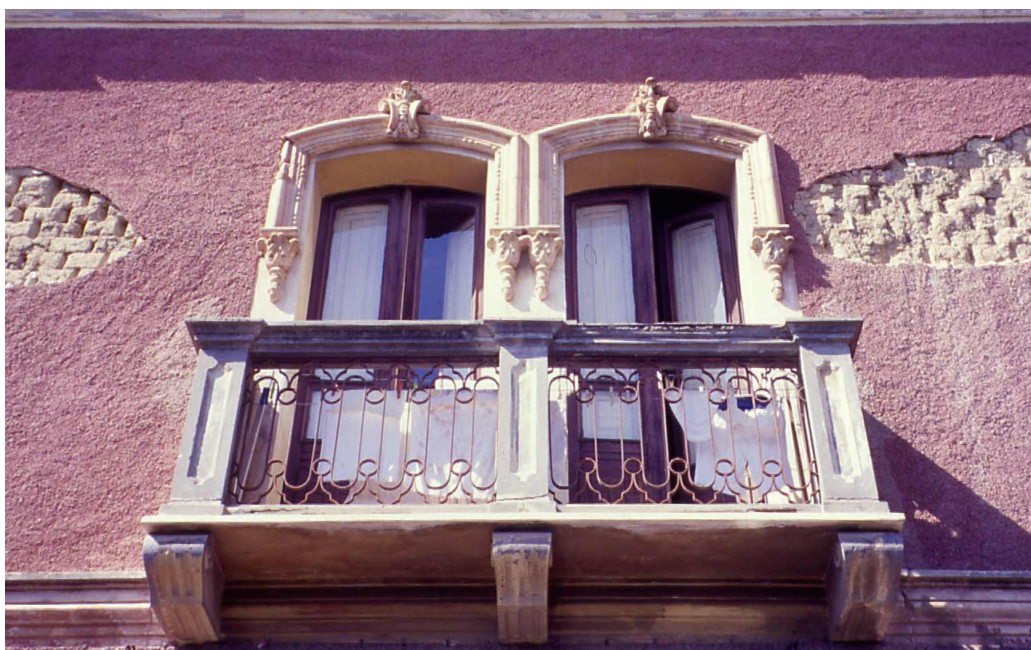
Fig. 1. An earthen building of Campidano showing lime render on mud brick masonry
