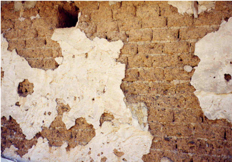
Fig. 2. Sampling of lime render was done to cause minimum destruction, and mostly in building with high decay levels such as this one in the village of Sinnai.
