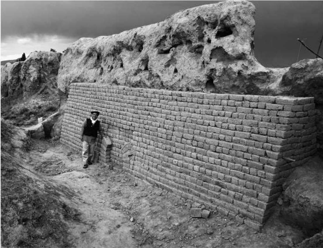
Fig. 13. An example of conservation work. Wall-B is supported by buttresses made of new mud bricks.
