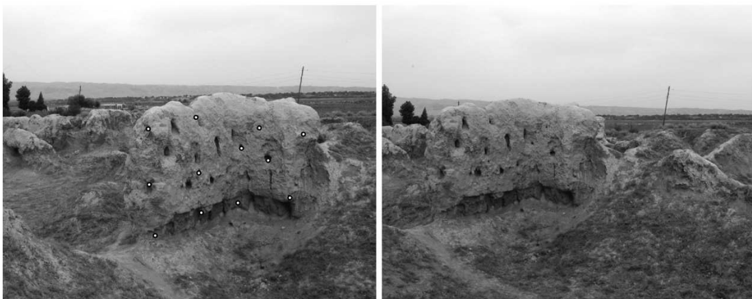
Fig. 2. A pair of stereo-photographs of a damaged wall (Wall A in Fig. 8). White circles on the left photograph show control points.
