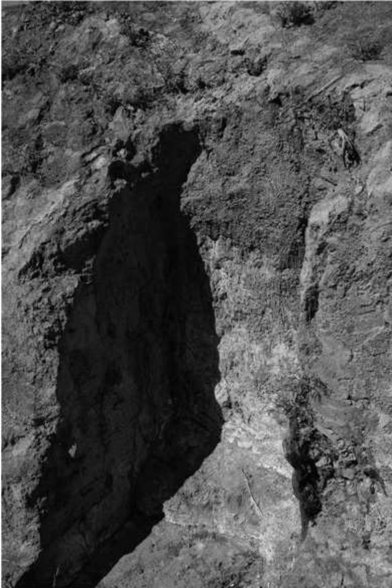
Fig. 12. Salt precipitation on an excavated surface of the building wall. The excavated height is about 1 m.
