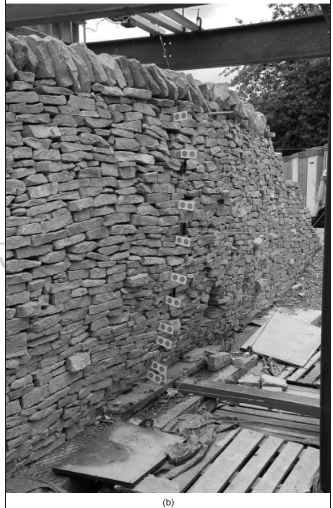
Figure 9. Test wall 3: (a) survey readings; (b) prior to failure
