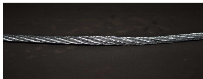
(a) The rope fatigue defect of the steel cord conveyor belt
