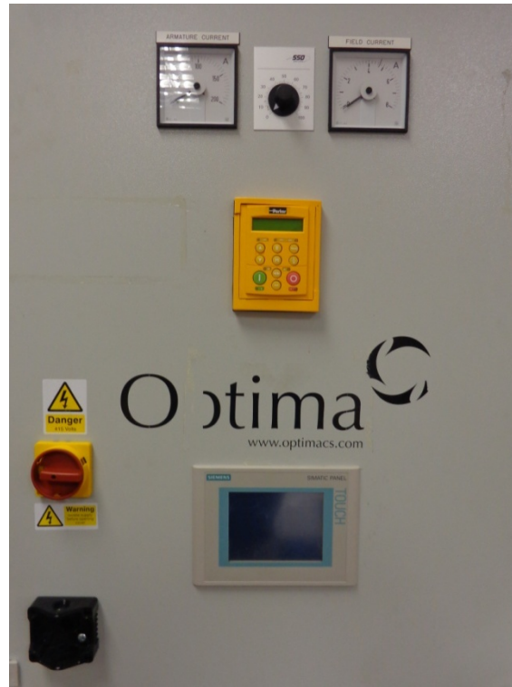
Figure 6.7 Test rig control panel
