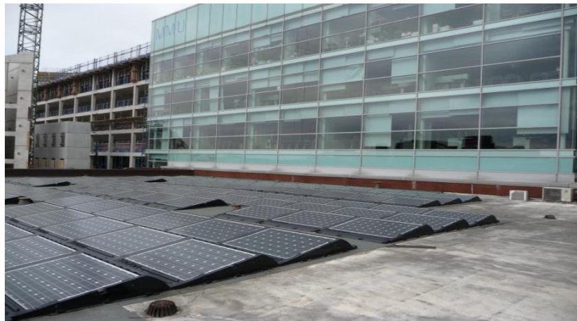
Figure 8.7 (a) All Saints building PV array 1
