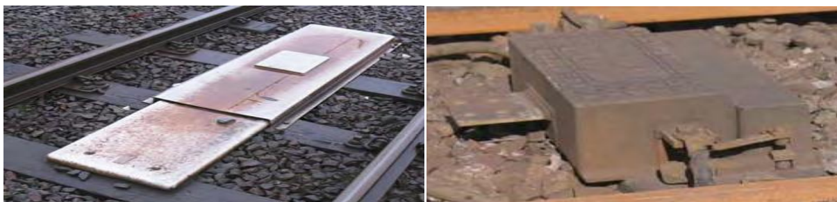
Figure 5.27 Photographs of VIS loop (left) and signalling apparatus (right) in situ. VIS loop indicates to signals and a control room the relative location of a vehicle on the network. Signalling apparatus is used to control and direct traffic around the network.
