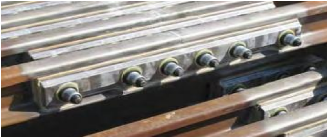
Figure 5.4 A photograph of pre-prepared insulated fishplate joint. An insulated fishplate joint allows two sections of track to be joined but remain electrically isolated.
