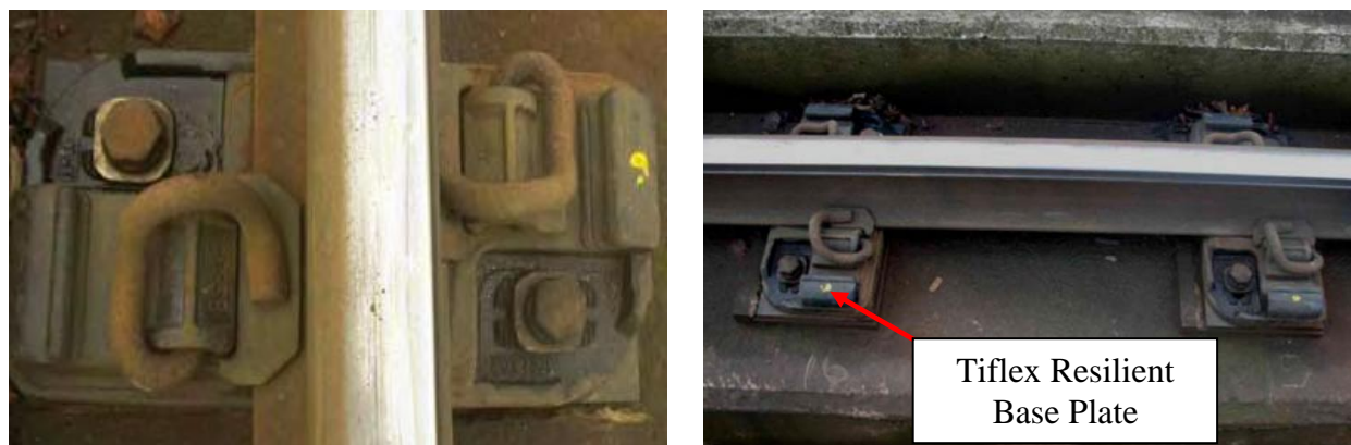
Figure 5.17 Photographs of Pandrol ‘e’ clips on a Tiflex resilient base plate in situ. A Pandrol clip secures rail in position while a Tiflex resilient base plate reduces ground born vibration in non-ballasted track areas.
