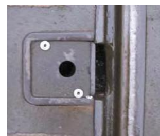
Figure 5.39 A Photograph of a drain gully catch pot for drainage of water.
