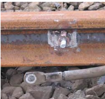
Figure 5.26 A photograph of a Broken cable attachment that provides a traction current return.
