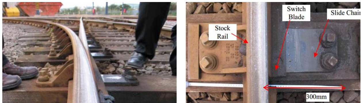
Figure 5.20 A switch blade on a variable slide chair mounting in situ, used to allow traffic to change lines.
