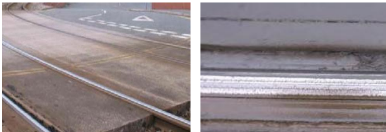
Figure 5.32 Photographs of Twin flange-planned for checkrail. This is used in small sections of embedded track where grooved rail would not be suited.
