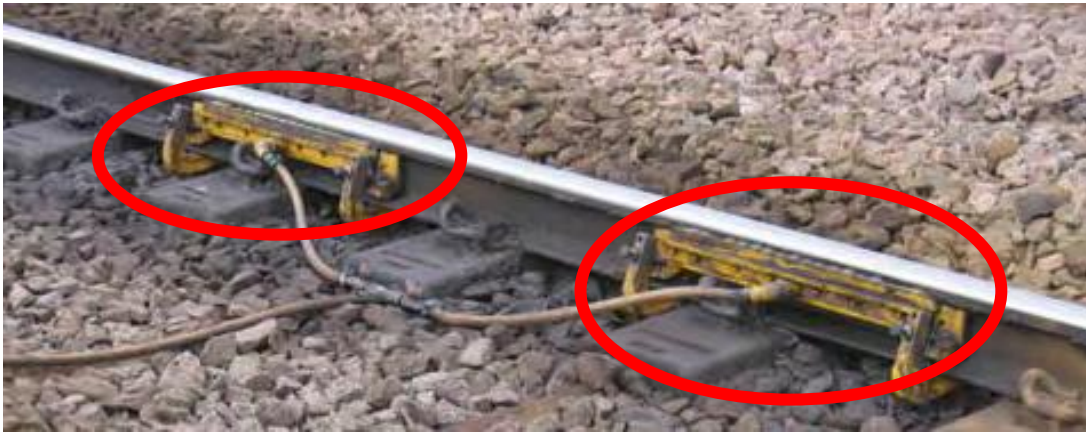
Figure 5.25 A photograph of Jumbo lubricators in situ. Lubrication is used to prevent excessive wear on curved track and prevent rolling contact fatigue occurring.
