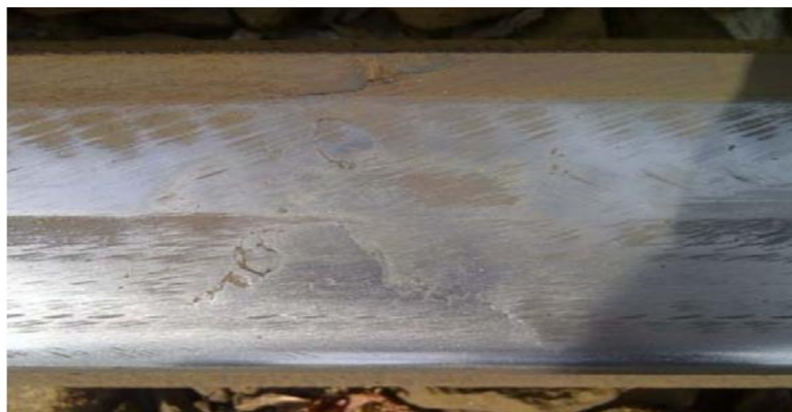
Figure 5.46 An example of a severe squat on the running surface of a flat bottom rail.
