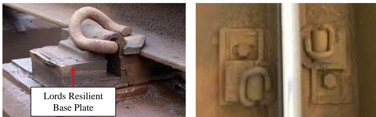
Figure 5.18 Photographs of Pandrol ‘e’ clips on Lords resilient base plates in situ. A Pandrol clip secures rail in position while a Lords resilient base plate provides noise dampening in urban environments.
