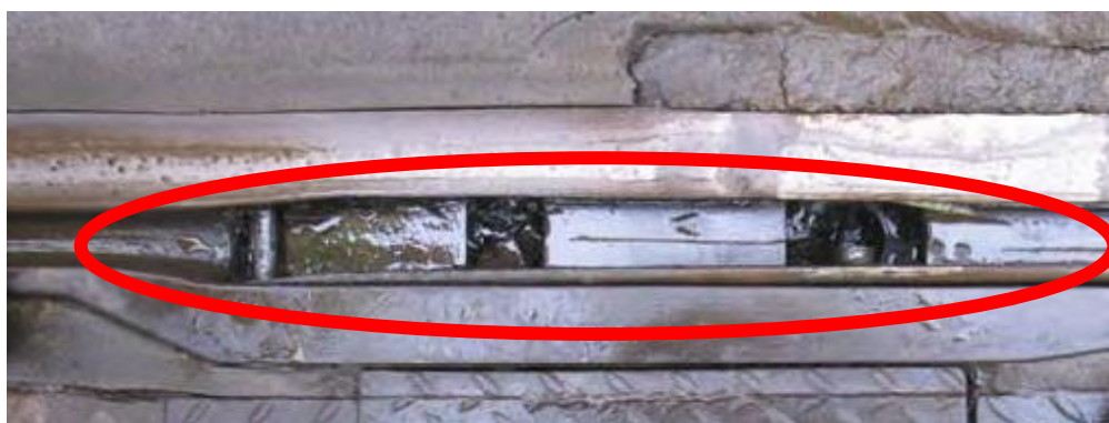
Figure 5.36 A photograph of an Embedded expansion joint. This allows lateral expansion of embedded rail due to weather.
