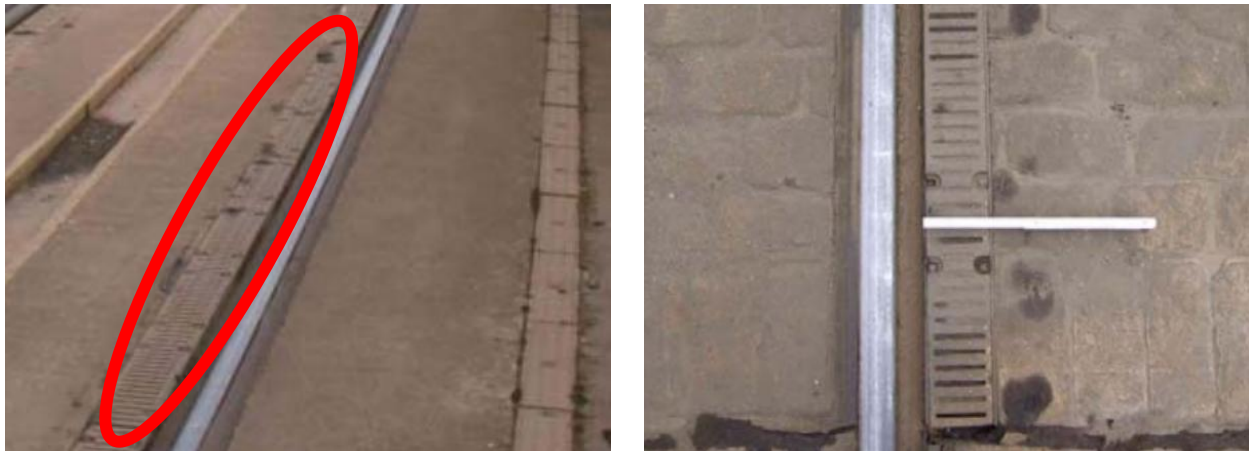
Figure 5.34 Photographs of adjacent flange-path Aco derailment channel. These are designed to aid in drainage and provide a path for a potential derailed wheelset to follow
