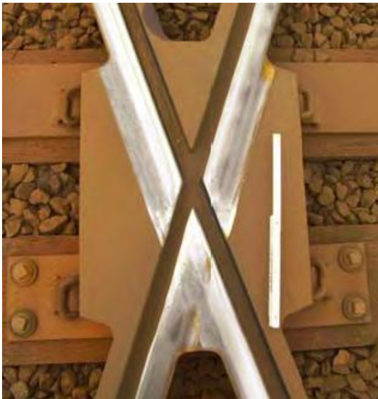
Figure 5.22 A photograph of a PR7 diamond mono block crossing in situ, used to allow traffic to cross lines.
