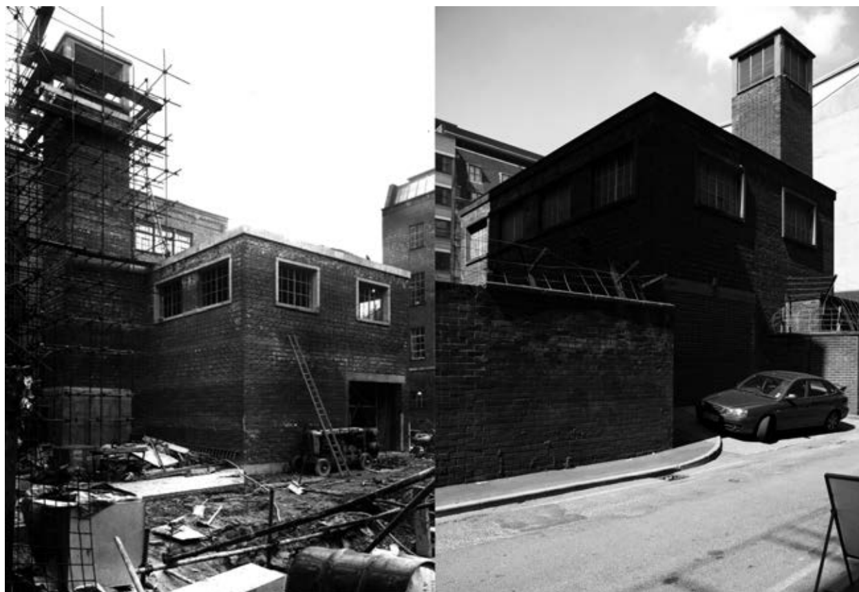
Figure 3. [image left] Original photograph documenting the construction of the service building at 56 George Street, Manchester, dated November 1960. Photograph taken inside the compound. The distinctive exhaust tower is nearly complete. (Source: Photograph by tunnel engineer Patrick Gough. Courtesy of George Coney.) [image right] A contemporary view of the utilitarian same building at the top of the main equipment lift shaft down to the GUTE . The compound now features significant physical perimeter security. Photograph taken from Back George Street (Source: Richard Brook).
