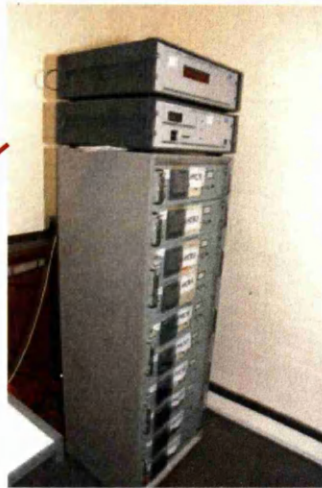
(furnace control unit)
