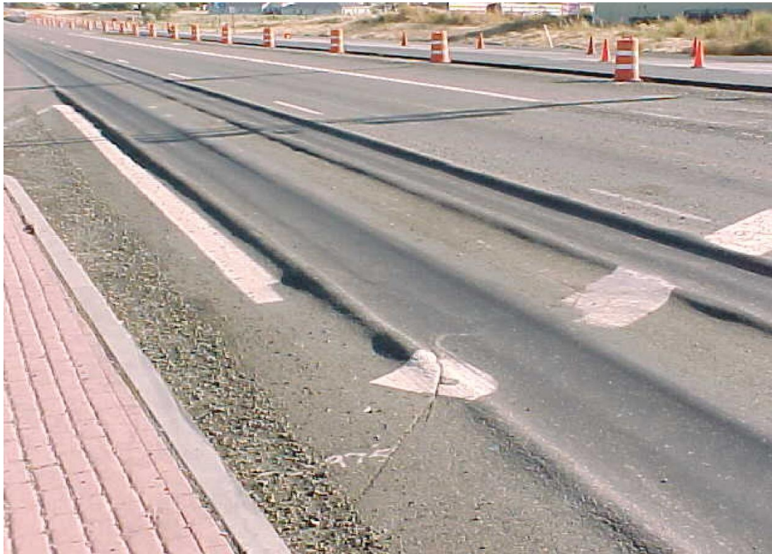
Figure 1.1: Rutting of bituminous pavements (Pavement Interactive, 2012)
