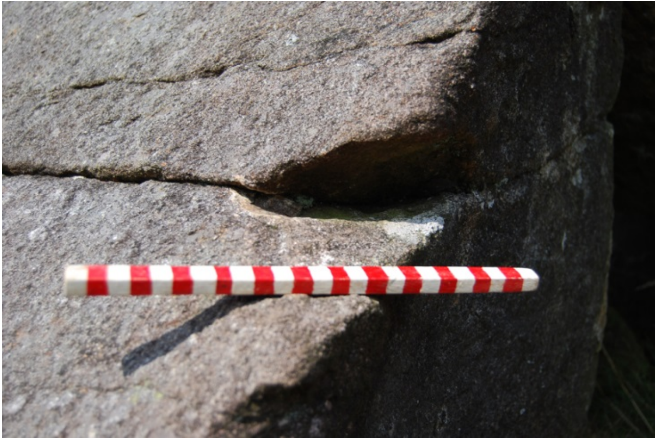
Figure 9. Widening of a joint between pillars at Carn Goedog, viewed from the south (photograph by Duncan Schlee).
