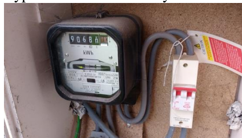
Typical Sangamo Weston Ltd. Electricity
