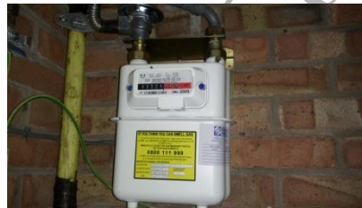
Typical George Wilson (new) make gas meter
