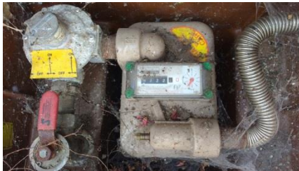
Typical schlumberger make gas meter
