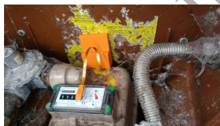
Gas metering in a typical house after Loop Energy device installation
