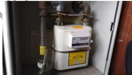
Typical Krome Schroeder gas meter
