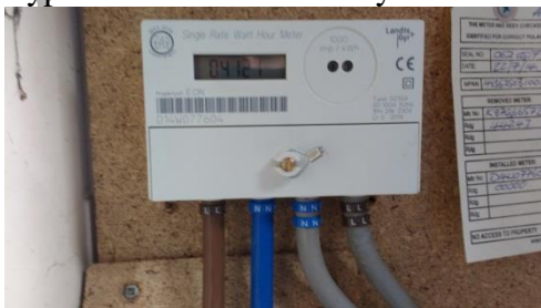
Typical Landis Electricity meter
