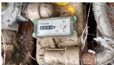
Gas metering in a typical house before Loop Energy device installation
