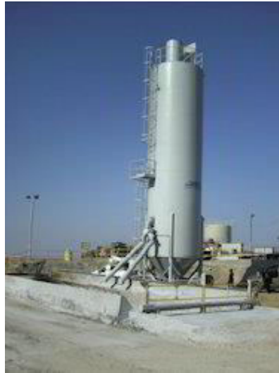
Figure 7 - Cement Storage Silo.
