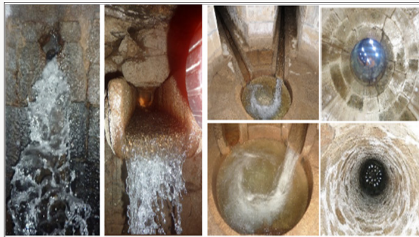
Figure 13: Water treatment processes performed inside the “chapels” (aeration, gas transfer, iron and manganese removal, sedimentation).
