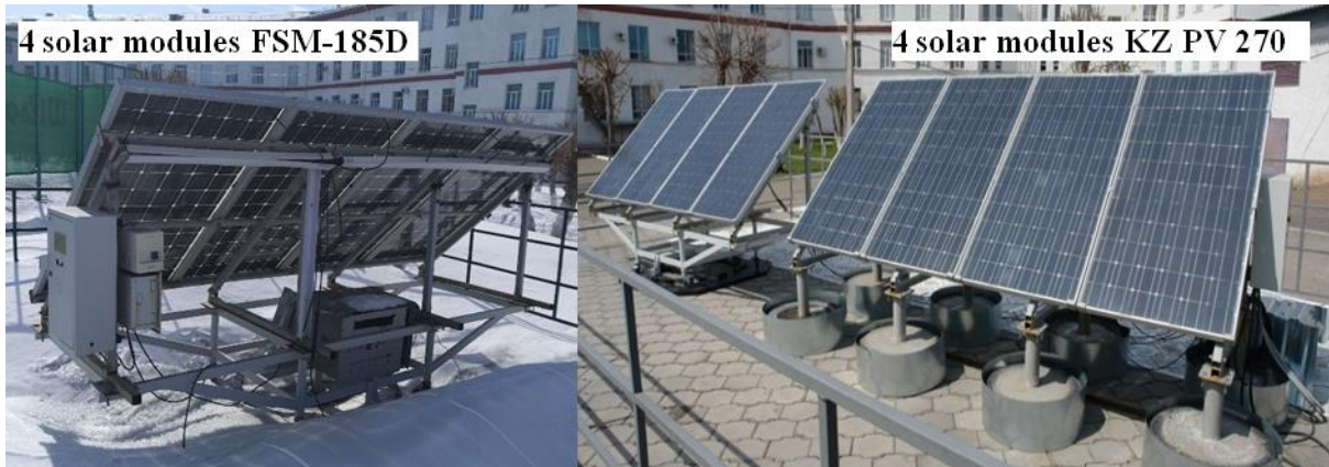
Fig. 1. External view of SPP with FSM-185D double-sided modules
