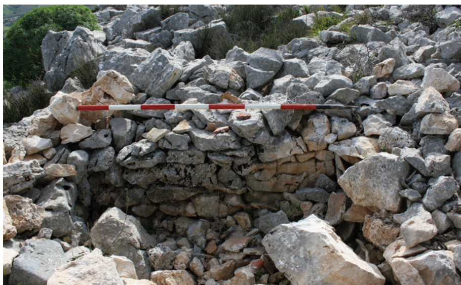
Fig. 11. Pizzo Monaco (Site O4 UT 01), internal wall of a cell and collapsed material.
