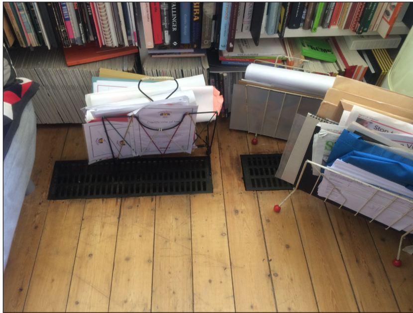
Figure 35: Floor grill covering underfloor radiator (perimeter) at upper floor.
