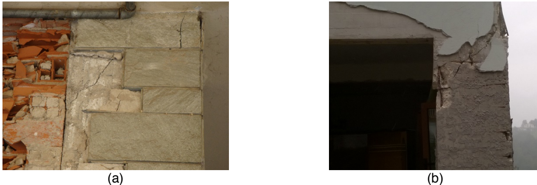
Figure 1. Column shear failure in RC infilled buildings in Italy (a) after the 2012 Emilia earthquake (Parisi et al. 2012) and (b) after the 2016 Central Italy earthquake (De Luca et al. 2017).
