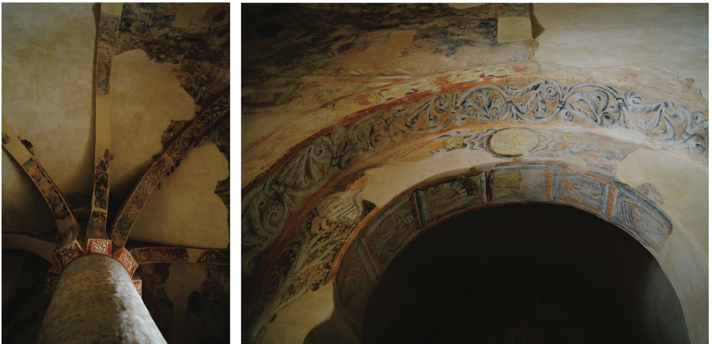
Left: The palm tree column, still decorated with historic paint, provides the structural support for the ceiling, Right: Decorative motifs still remain on the archway of the apse. Images: Author
