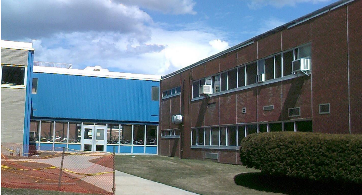
Figure 18. Damage to Bedford High School by Hurricane Sandy.
