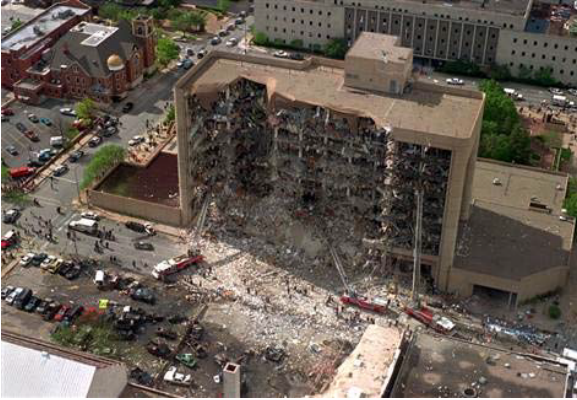
(a) Collapse of the 9-story Alfred P. Murrah Federal Building in Oklahoma City (1995)
