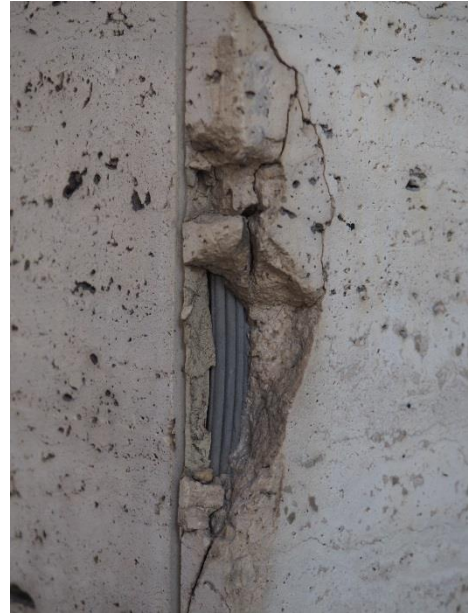
Figure 4.11 Juilliard School – Travertine Spall
