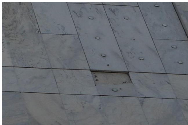
Figure 5.12 Exterior Deterioration – Delamination of Marble from Concrete
