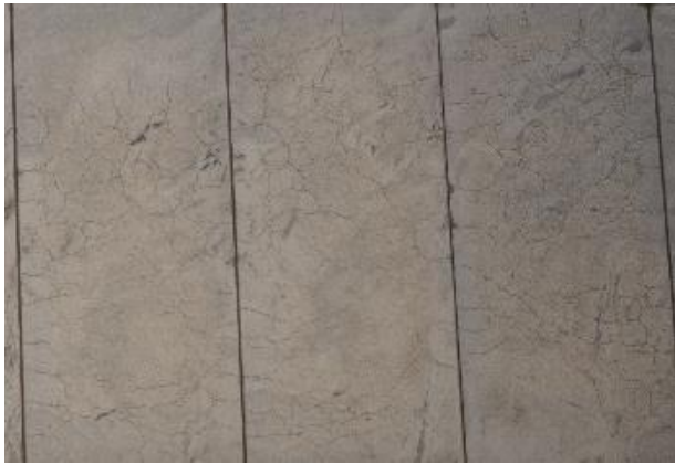
Figure 4.14 Former Life of Georgia Tower – Flexural Cracking
