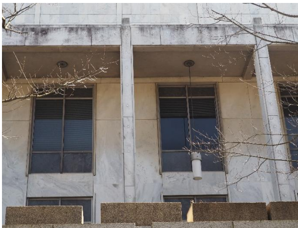
Figure 5.6 Exterior Deterioration – Soiling
