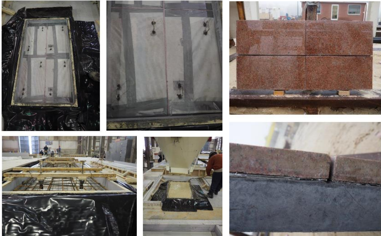
Figure 3.7 Gate Precast Demonstration: a.) stone and bondbreaker in wood mold b.) anchors and epoxy c.) secured rebar d.) pouring of concrete e.) finished panel surface with red granite f.) side view of precast concrete, bondbreaker, and granite
