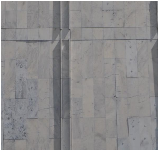
Figure 5.8 Exterior Deterioration – Horizontal Cracking
