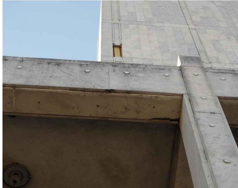
Figure 5.10 Exterior Deterioration – Missing Marble Fin and Bolting Repairs
