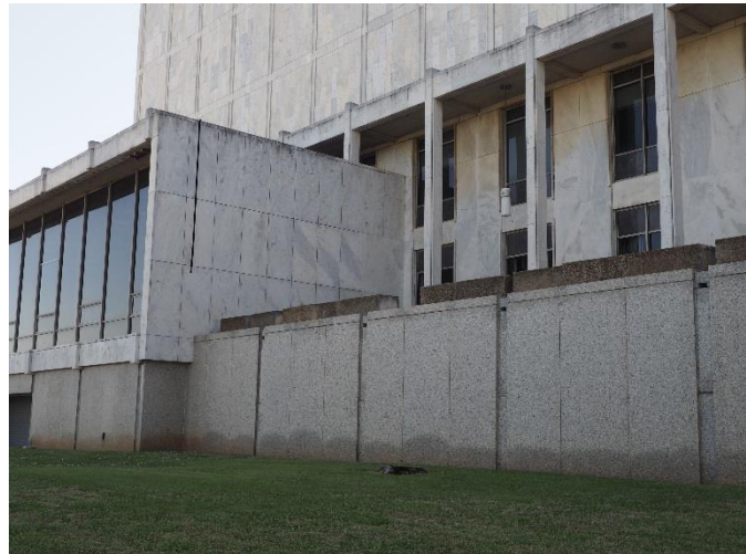
Figure 5.9 Exterior Deterioration – Moisture in Foundation
