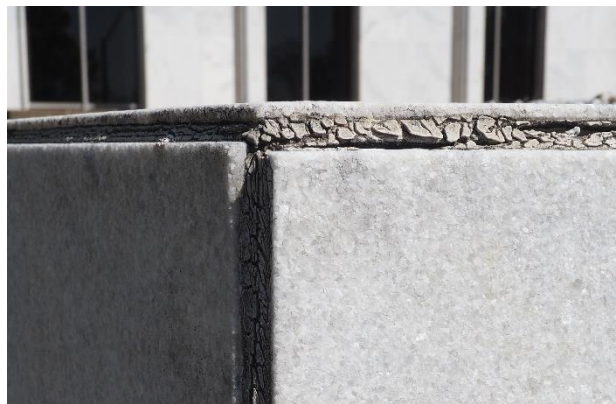
Figure 5.11 Exterior Deterioration – Moisture in Foundation
