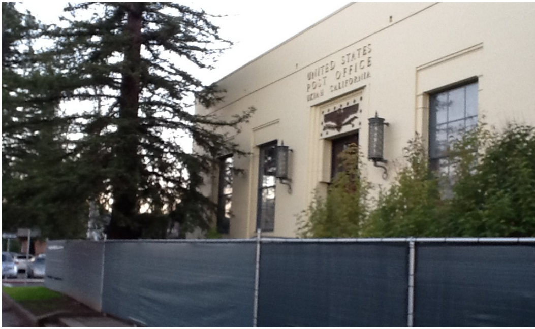
Image 26. Ukiah Post Office, condition as of early 2016. Image courtesy of Jacquelyn McCormick.
