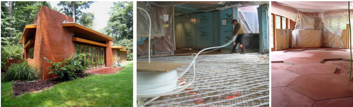
Fig. 31 – Restoration of the radiant heat system and the concrete mat floor in the Usonian Richardson House, designed by Wright in 1941 and built in 1951. (Source: Tarantino Architects)
