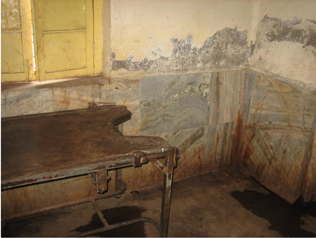
VII. CHC Rehali district Sagar, Madhya Pradesh February 2009 CHC labor room with old, rusted equipment even though untied funds are unspent.
