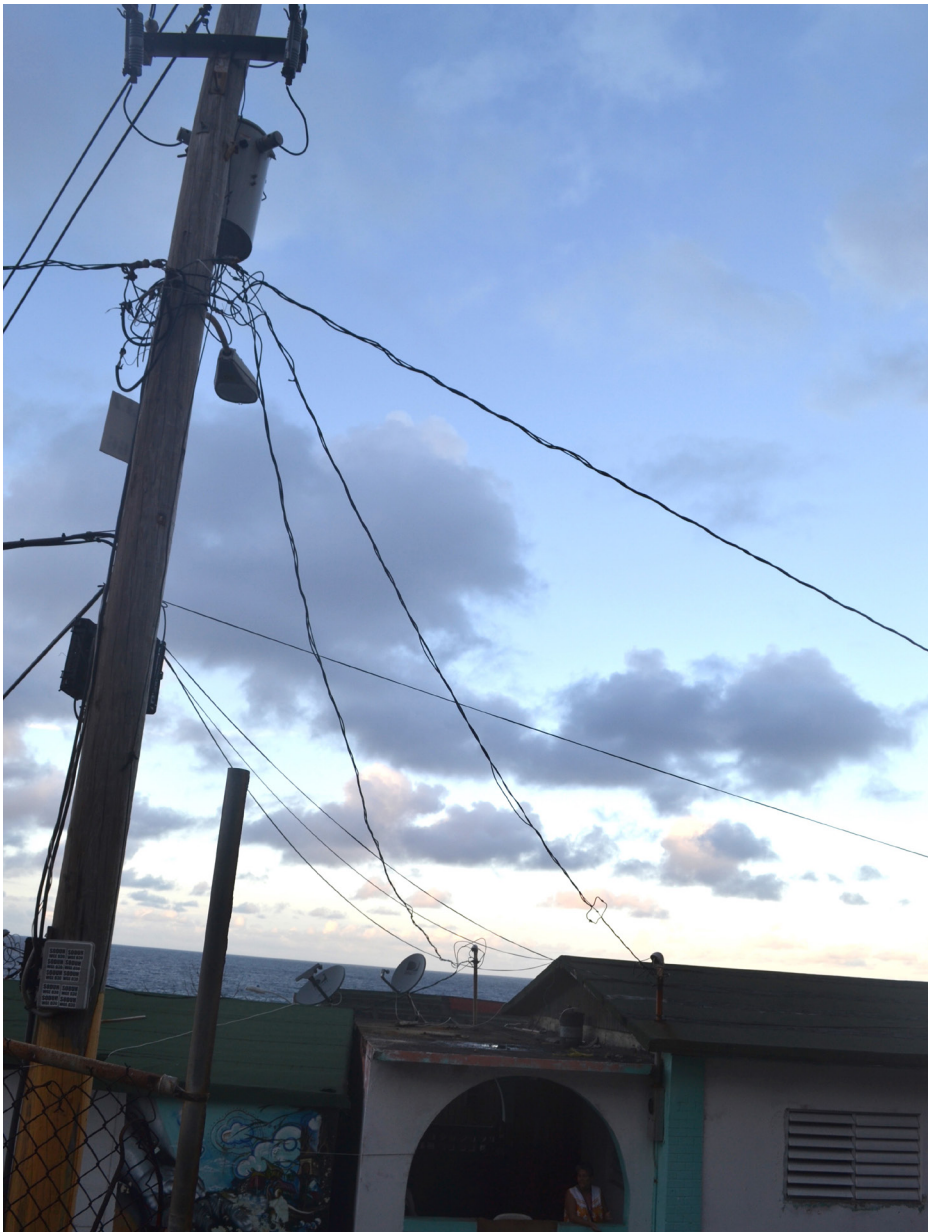
Figure 28. House in La Perla connected directly to a lamppost.
