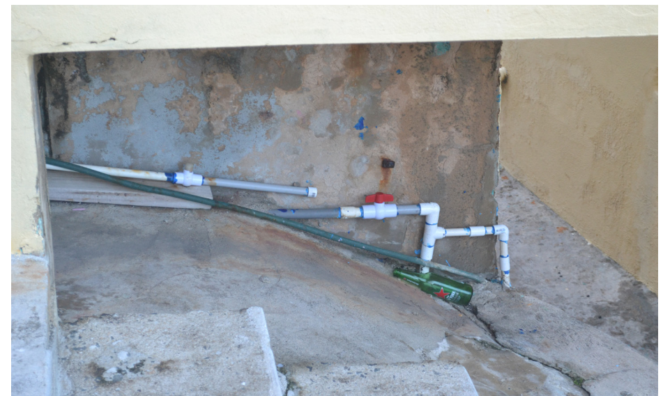
Figure 30. Makeshift water connections.
