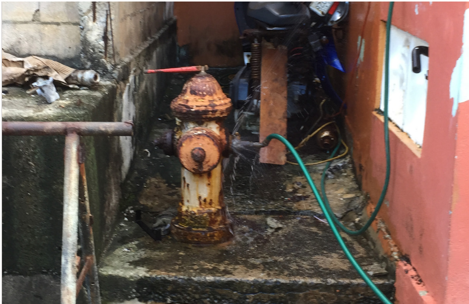
Figure 39. A fire hydrant in La Perla
