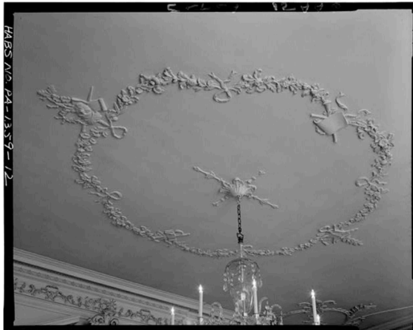
Figure 4.3: Detail of the reproduction of the “ballroom” ceiling at the Powel House. Source: Historic American Building Survey, 1967.
