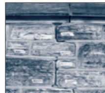
INTERIOR WATER DAMAGE
