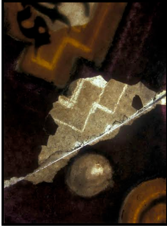
Figure 56. Example of enamel loss due to a problem with the coefficient of expansion of the glass and/or the enamel. Image courtesy of Drew Anderson.
