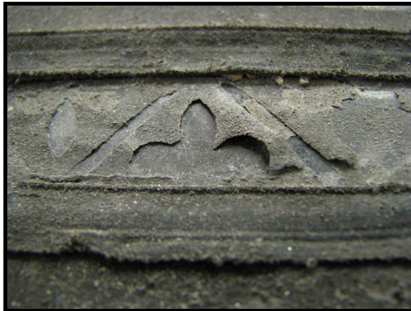
Figure 47. Flaking paint. Image courtesy of Drew Anderson.
