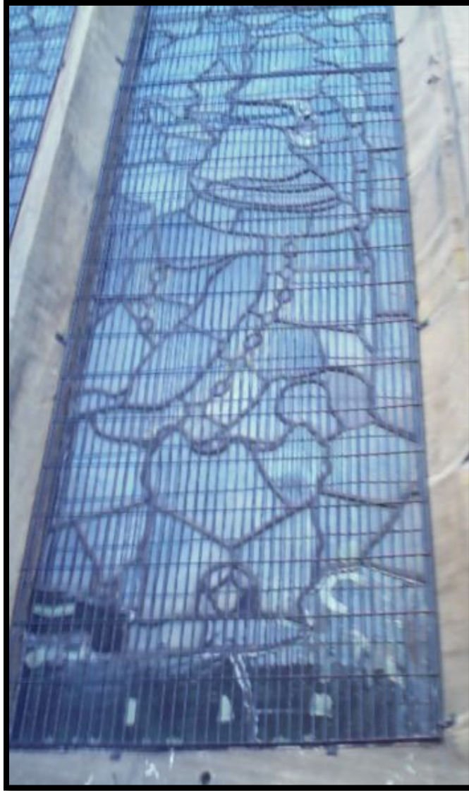
Figure 65. Wire guards used to protect stained glass windows. Image from http://www.abbestainedglass.co.uk/protection/wire-guards
