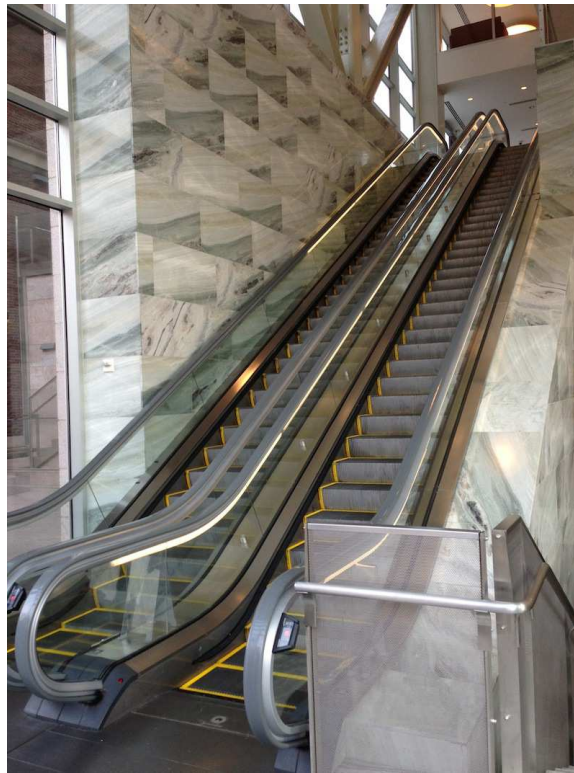
Figure 5.18: Escalator in Northwest Corner Building used for evaluation.
