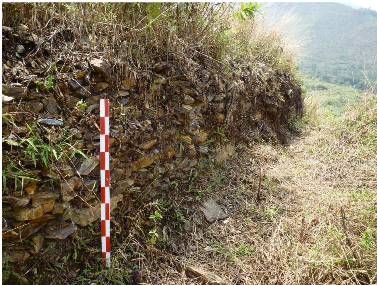
Figure 4.9. The retaining wall of the architectural terrace that abuts S-074, seen looking towards the east. Note the unfaced wall surface in comparison with the residential structures.
