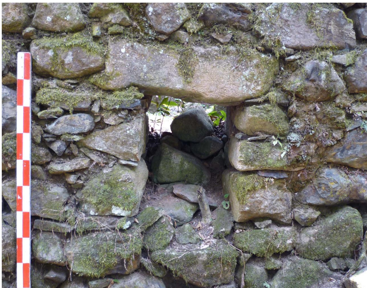
Figure 4.13. The drainage aperture in the eastern wall of S-004 (seen from the exterior of the structure).
