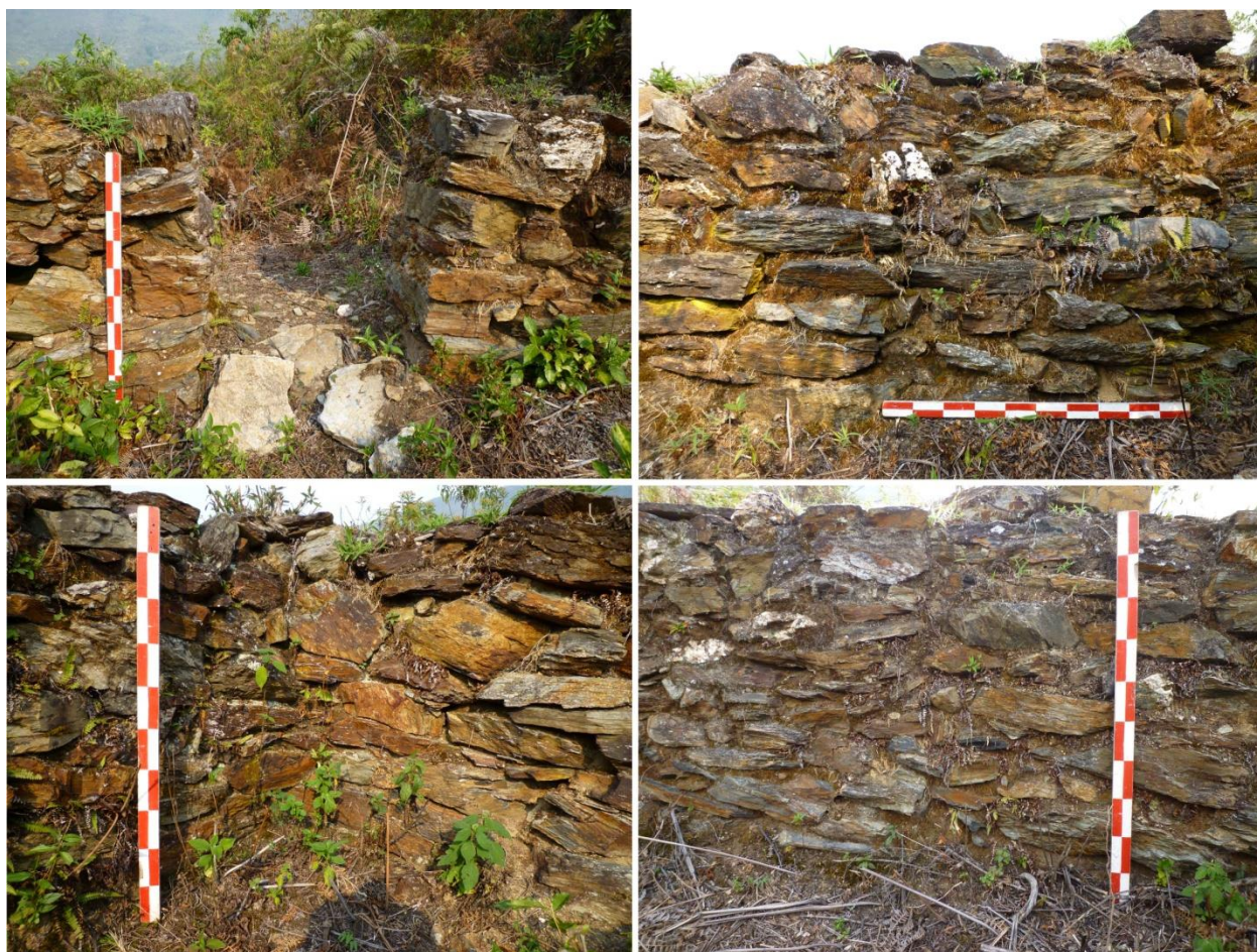
Figure 7.3. Photographs indicating typical entranceway construction (upper left), interior corner masonry (lower left) and interior wall masonry (upper and lower right) in building-type structures at Qochapata.
