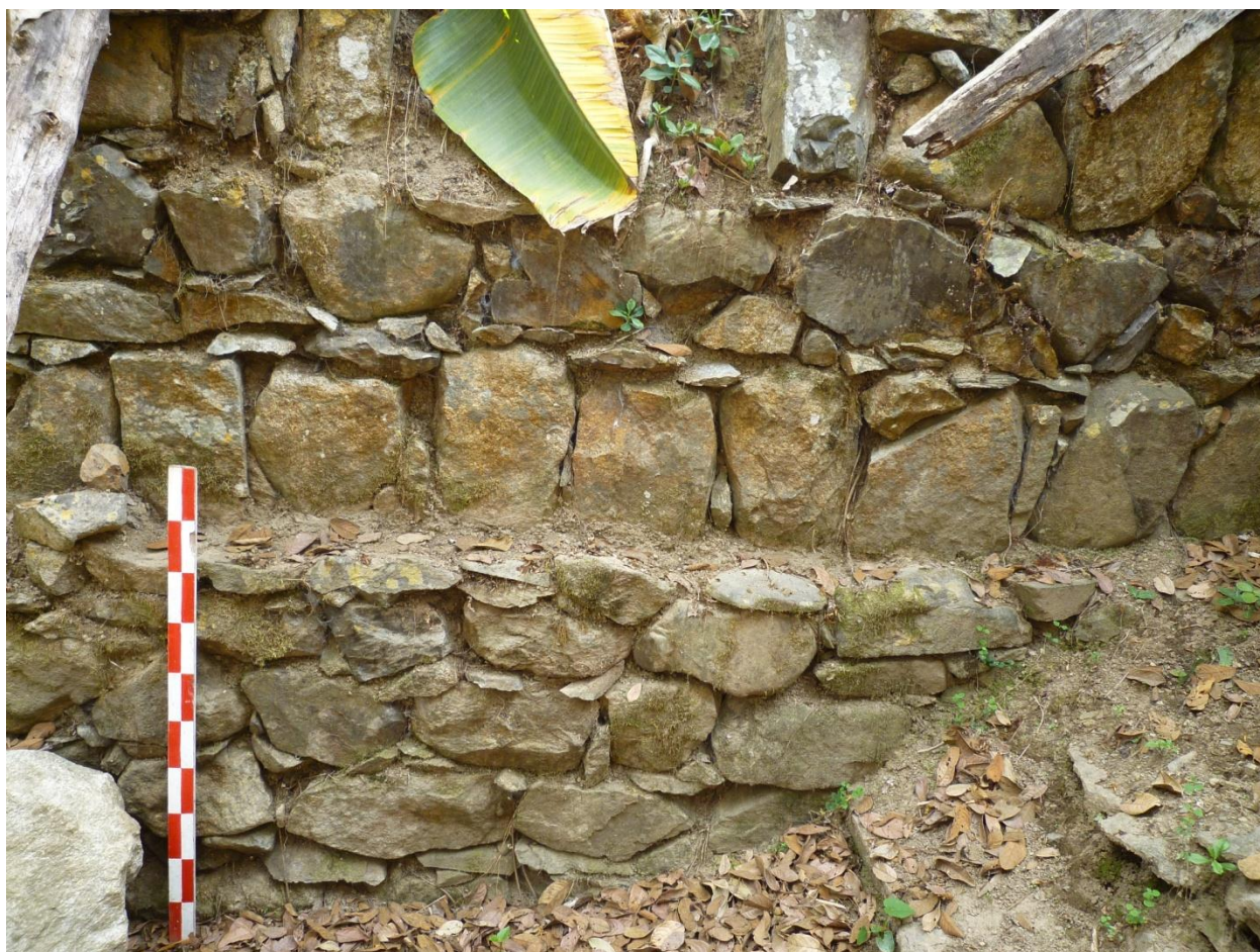
Figure 4.11. Interior wall face of S-001, seen looking west. Note the patterned masonry and the extruding ledge below it.
