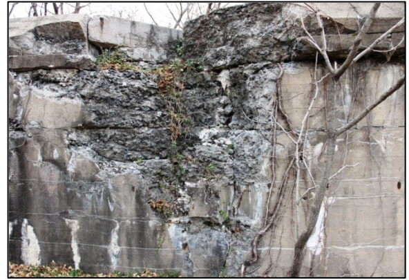
Figure 60: Freeze/thaw, calcite deposition and lateral movement of portland cement concrete in Battery Mahan 1 (2013)
