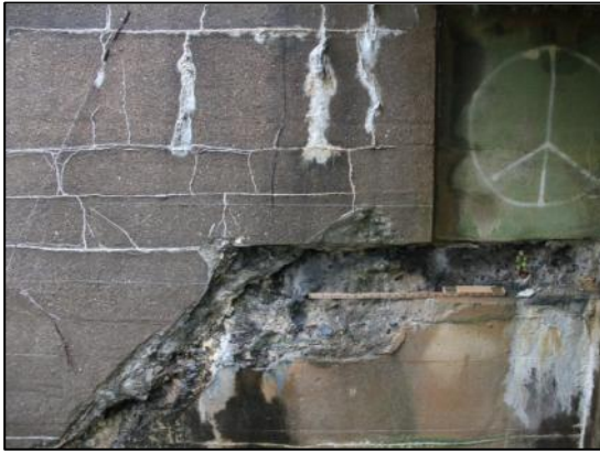
Figure 59: Battery Mahan 1, damage caused at the horizontal lifts (2013)
