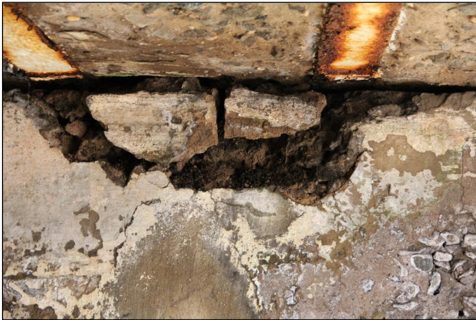
Figure 97: The gun emplacement foundations of Battery Graham 1 (1882-1897) with a slag cement coating
