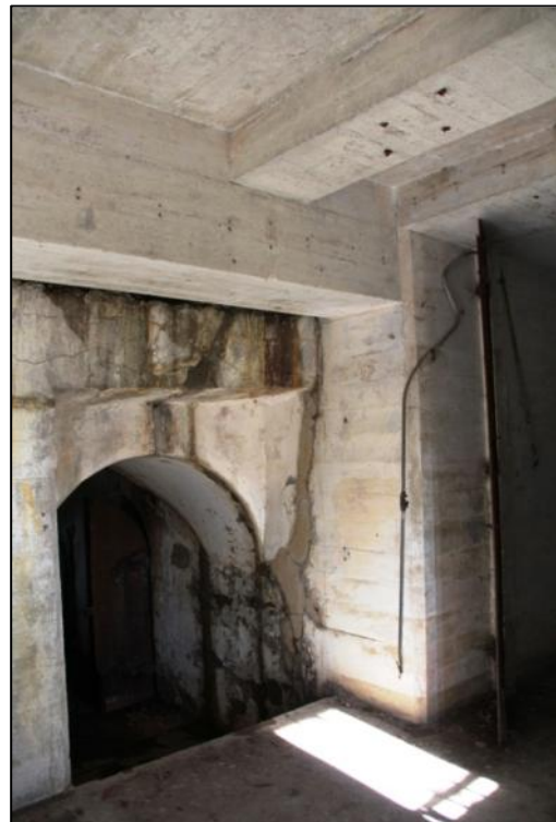
Figure 58: Battery Graham 1 showing the entrance to the original cast-in-place mass concrete magazines and the reinforced concrete columns and beams of the later extension (2012).
