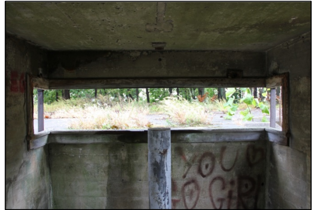
Figure 67: Base End Station on Battery Mahan 1, view of channel now obscured by trees and shrubs(2012)
