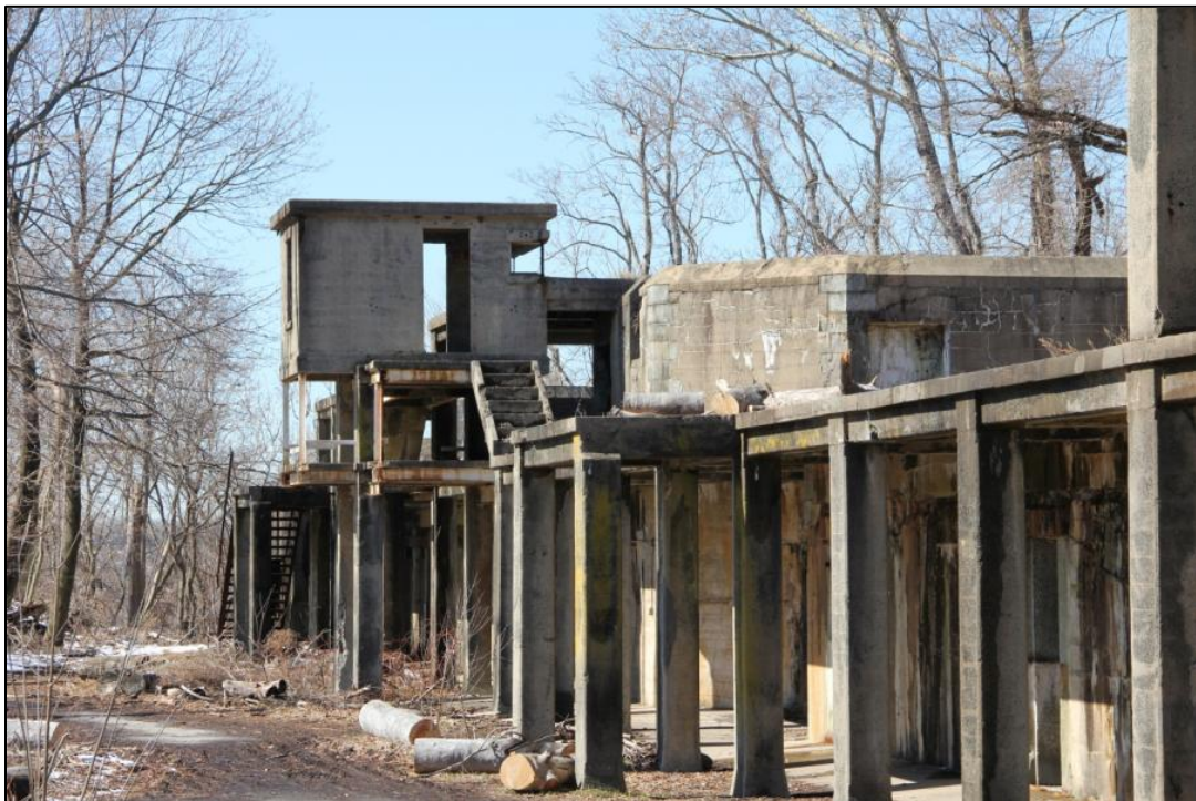
Figure 54: Battery Mahan 2 showing the later reinforced concrete extensions on the left and the cast-in-place mass concrete of the original traverses and magazines on the right (2013)
