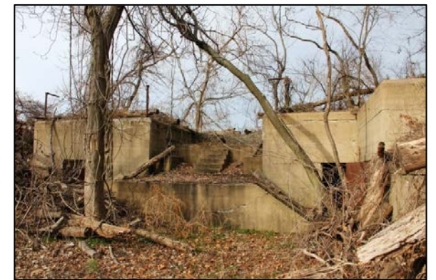
Figure 71: Battery Stuart, showing encroachment of trees and shrubs (2012)
