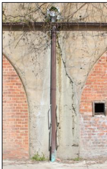
Figure 63: Crack between Torpedo Magazines 1 and 2 (2012)
