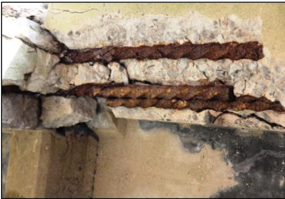
Figure 61: Failure of the reinforced concrete at the extensions of Battery Sumner 1 (2012)
