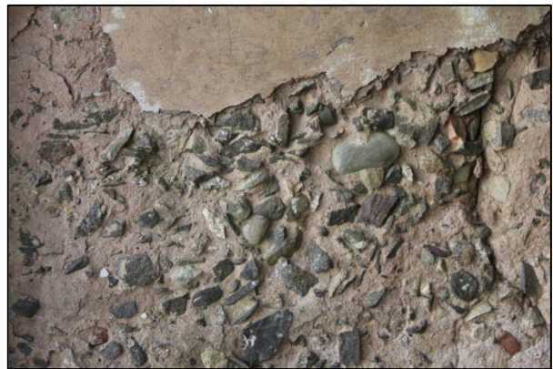
Figure 75: Exposed concrete showing large unbroken gravel aggregate in the Tunnel (1870-1871)
