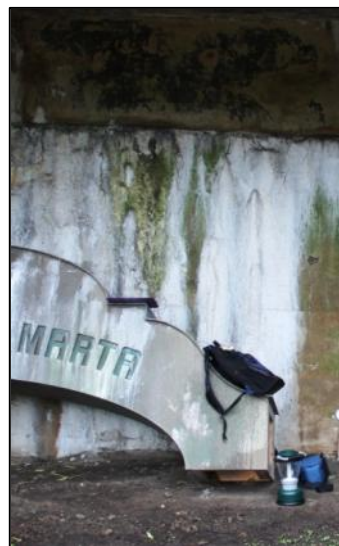
Figure 64: Horizontal cracking just below the second level at Battery Graham 1 with calcium deposits (2012)
