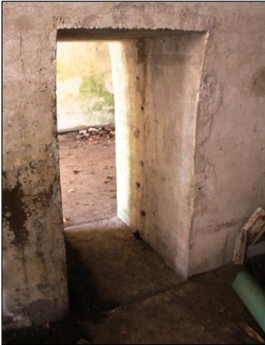
Figure 55: Torpedo Magazines, later doorway cut through the 4 feet thick dividing walls showing the mass concrete construction (2013)
