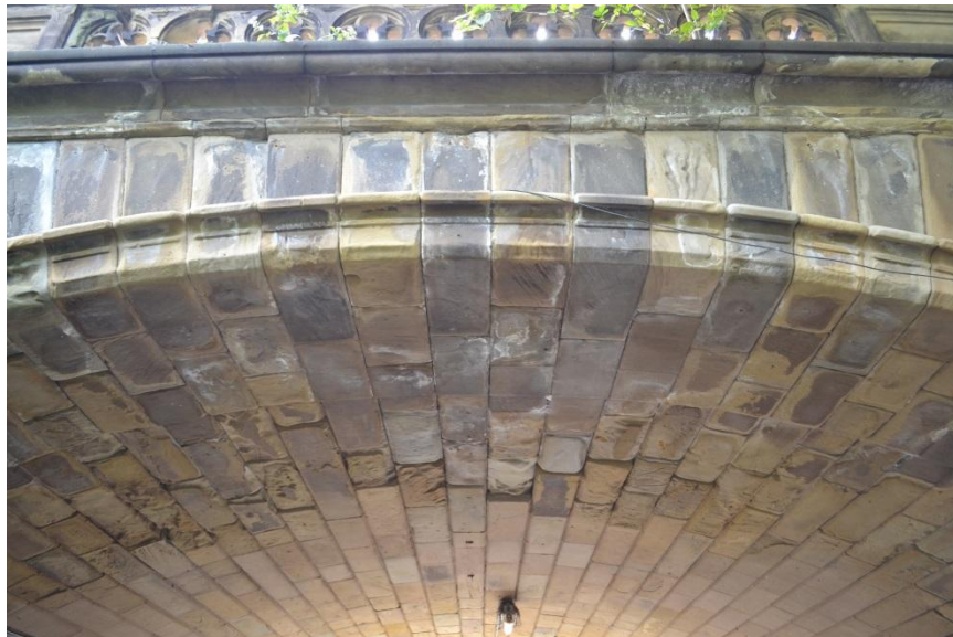
Figure 1.14: Denesmouth Arch showing deterioration conditions
