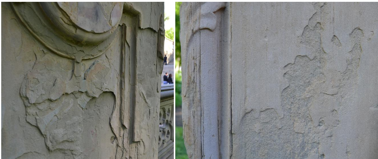
Figure 5.1: Bethesda Terrace pier deteriorating through exfoliation on one side and flaking on the other side
