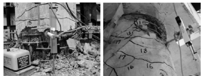
Fig. 3. Damage observed on the lower and upper portions of Bent-3 after T-19
