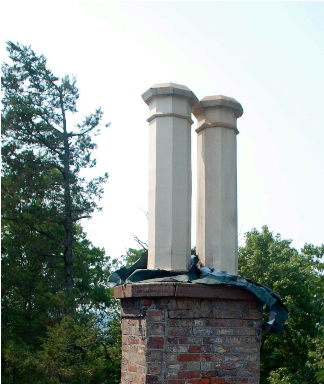
Dr. Oliver Bronson House. Detail of chimney post, N.E. chimney. Peter Watson.
