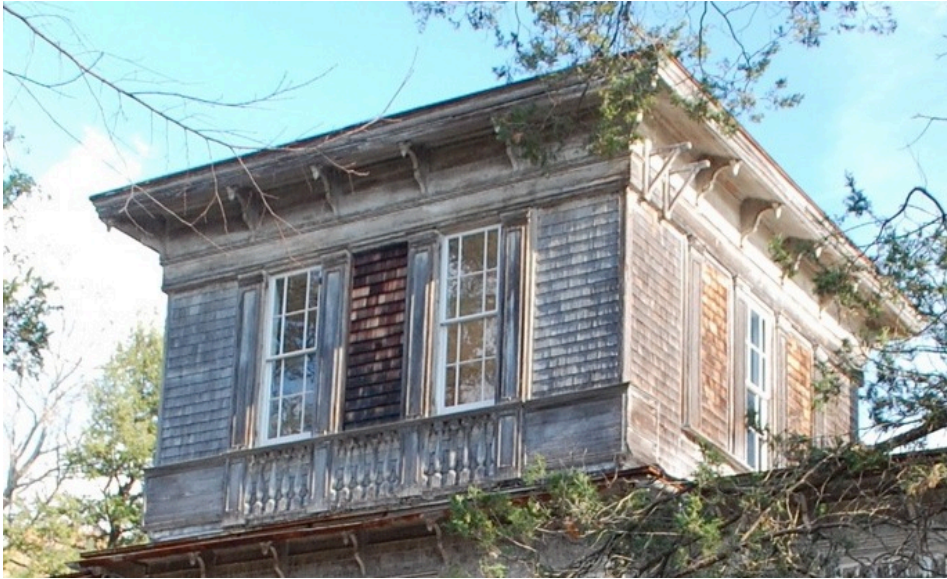
Dr. Oliver Bronson House. Detail of prospect tower fenestration showing location of original blind jalousies now covered over with shingles. Peter Watson.
