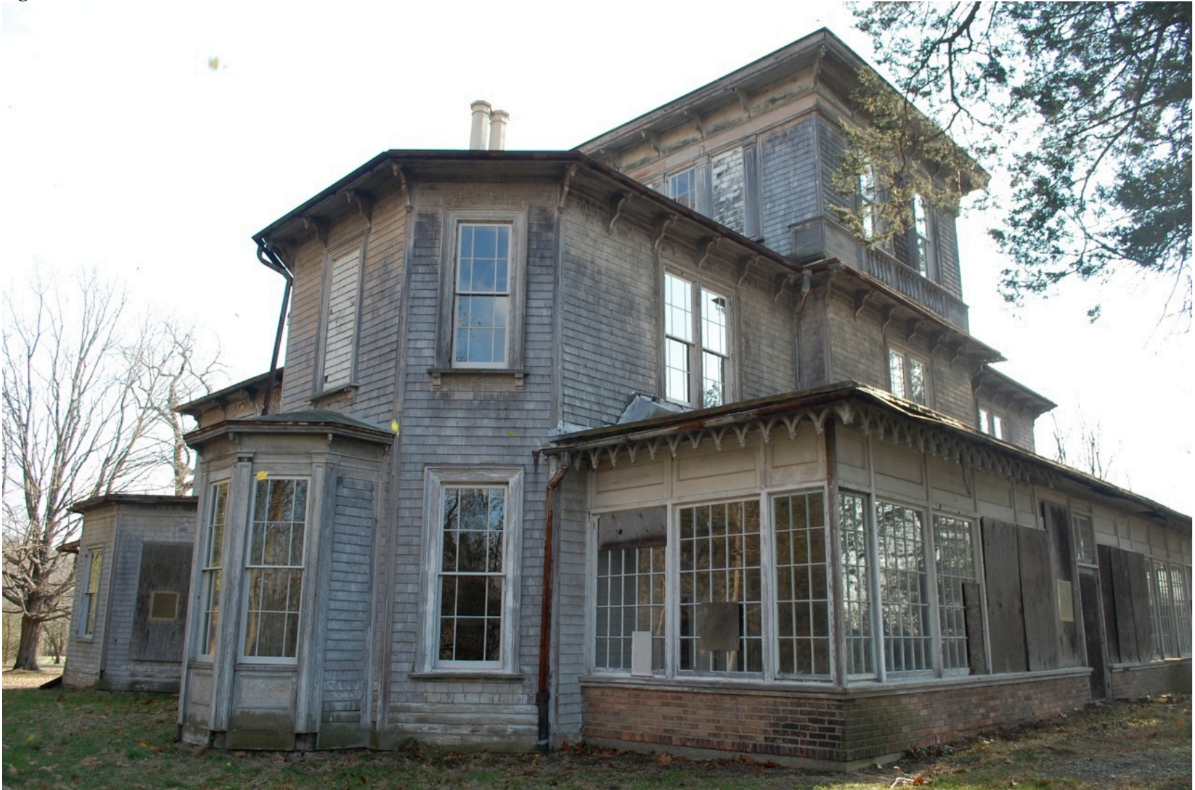
Dr. Oliver Bronson House. View of one-story northwest secondary bay. Peter Watson.
