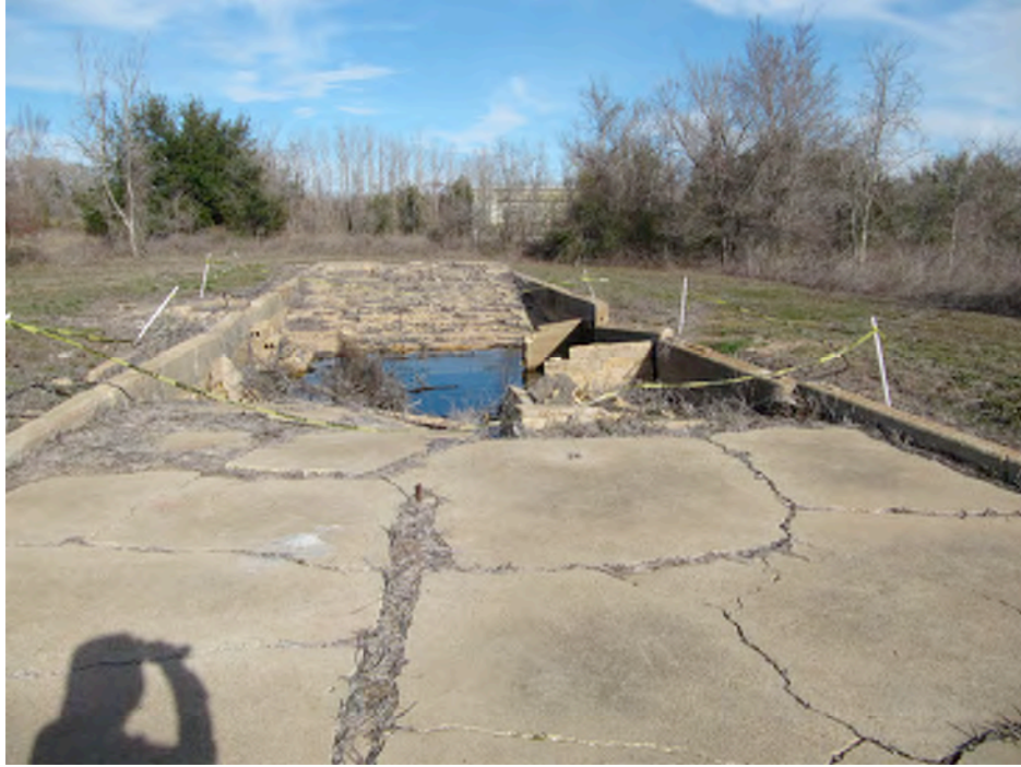
Figure 2-12: Remnants of the concrete foundation of the POW-built theater, with stadium seating visible in the back of the building (Rebecca Salgado)
